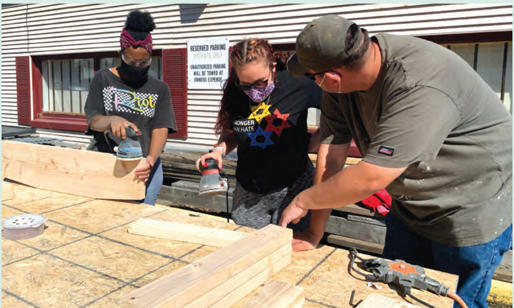
Johnstown Youth Corps members spent the summer making improvements around the city and constructing beds for kids who need them.
